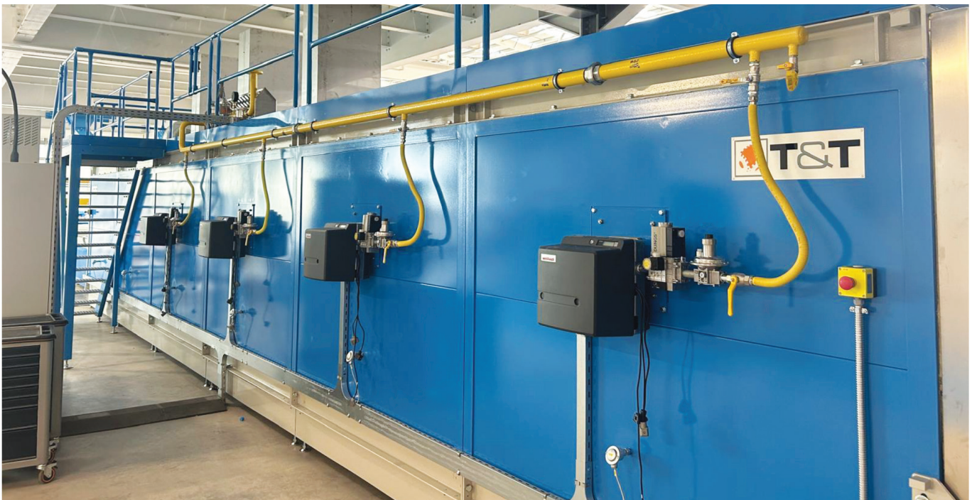
▲ Gas burners and access stairs to top of the lehr with safety rails for when working on top of the lehr.
